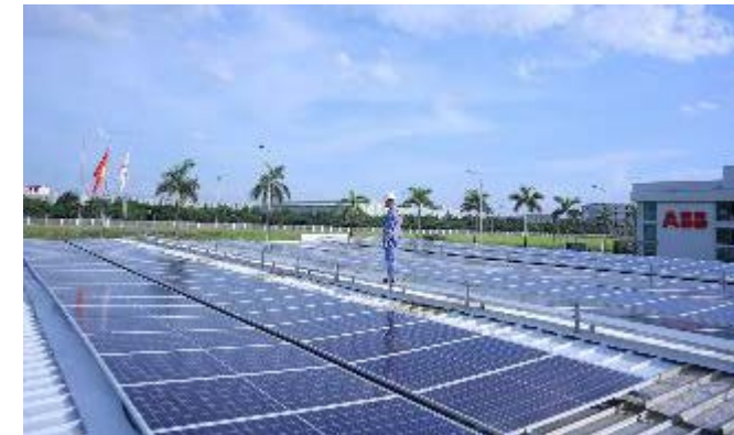
ABB Bac Ninh Factory 75 kWp (2018)
