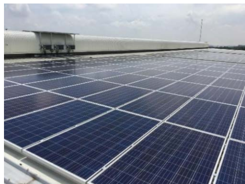
Emergent Cold Storage, Bac Ninh, 308 kWp (2016)
